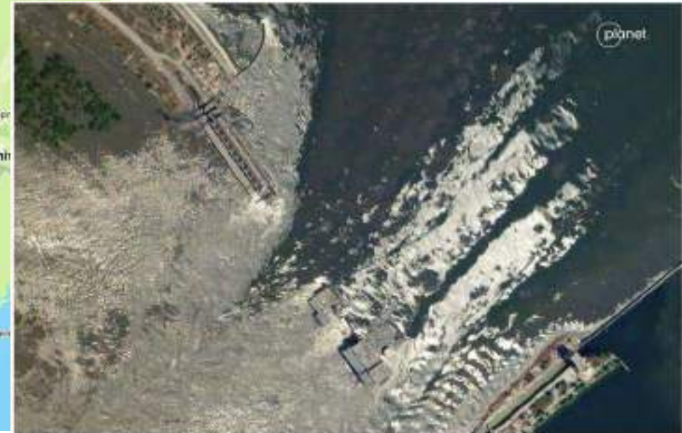
Figure 3. Satellite image shows the Nova Kakhovka dam breached (Image from Skywet courtesy of © 2023 Planet Labs PBC, available under a Creative Commons BY-NC 2.0 license at https://www.planet.com/gallery/#/post/destruction-of-the-kakhovka-dam )
